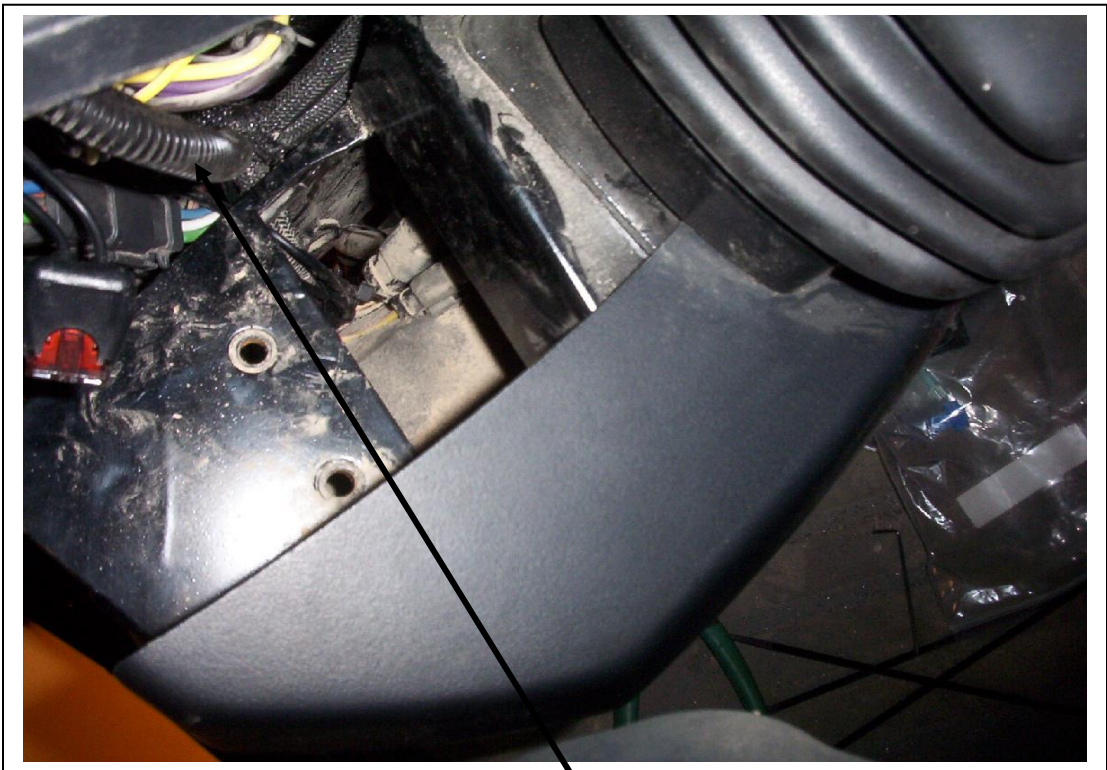
Clutch wire and thermostat probe going down and out of the cab through the floor to the drier and the evaporator.
